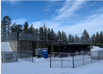
Above: Jean Road pump station
